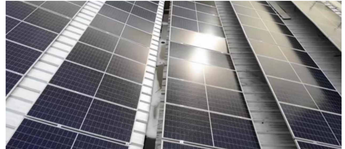
Solar photovoltaic panels of Zhenjiang warehouse
