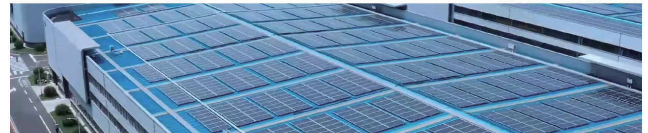
▲ Solar panels on the roof
