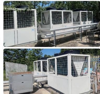
Air energy heat pump ▶
