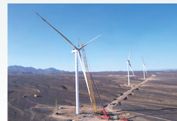
► Crawler cranes of Huaxia Financial Leasing are used for hoisting in the CSSC-Hami project
