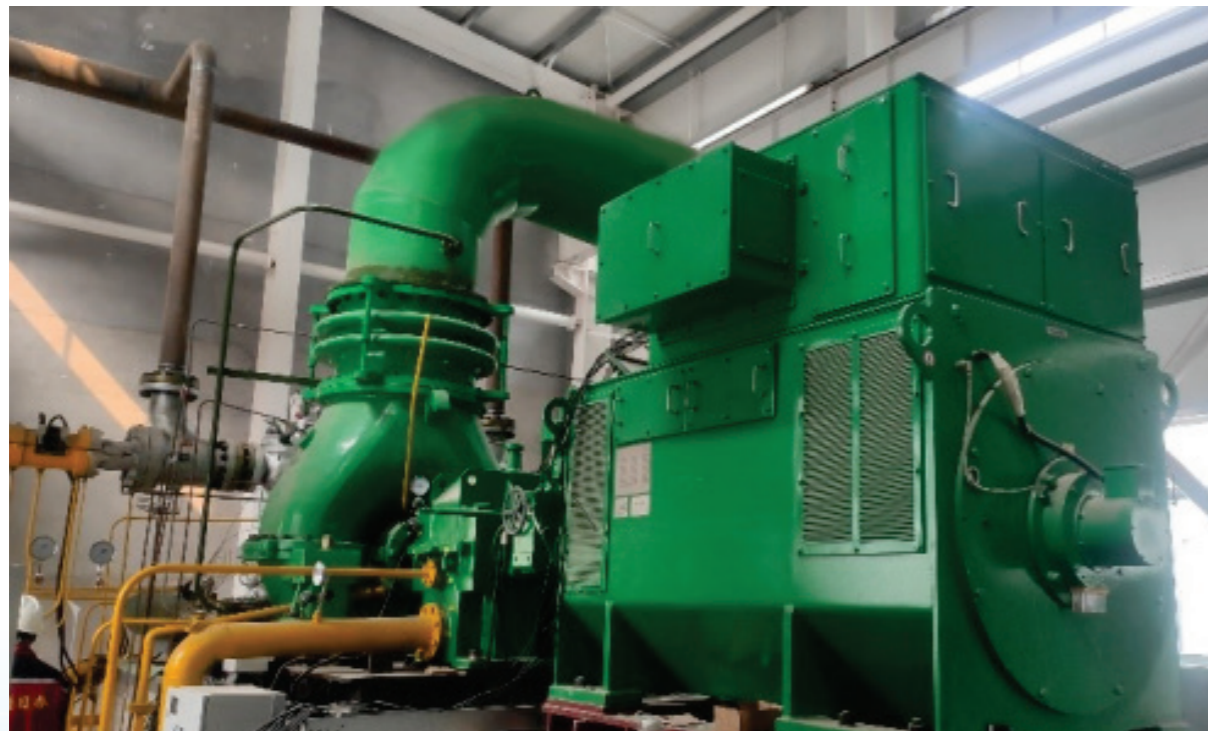
Waste heat turbine generator
