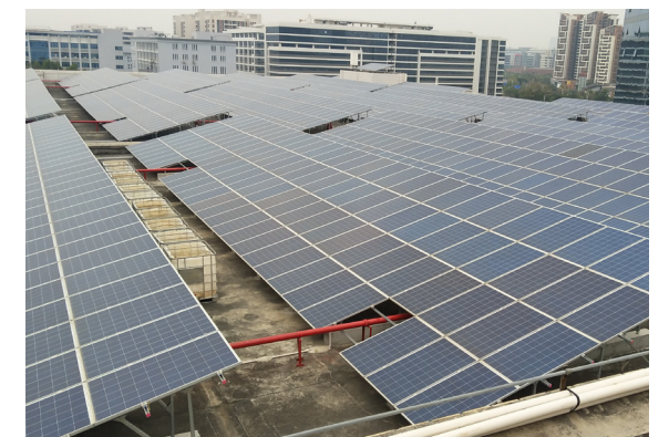
^ Rooftop Photovoltaic Site
