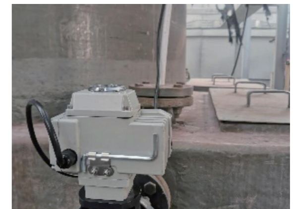
After modification - automatic valve
