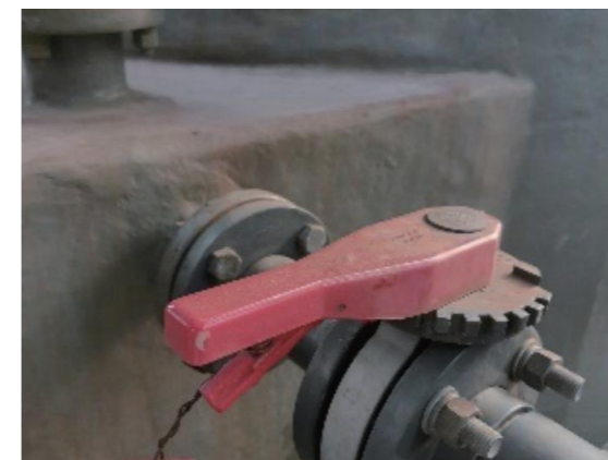
Before modification - manual valve
