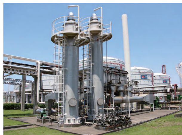
Organic Waste Gas Treatment Facilities
