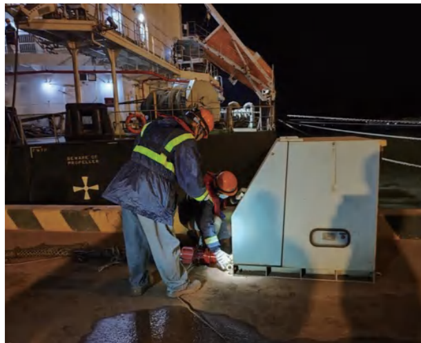
The "Baohang 58" vessel at Berth 1 of Taicang Wugang Terminal successfully connected to high-voltage shore power.
