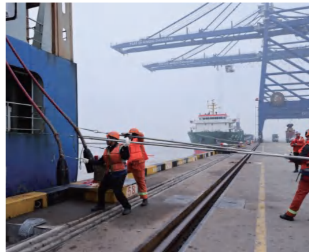
The High-voltage Shore Power at Daxie Terminal Was Officially Put into Operation.
